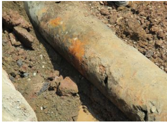
water main break
