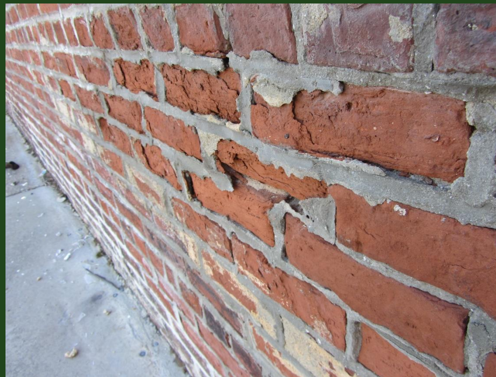
Hard Portland cement mortar is causing these historic bricks to spall
