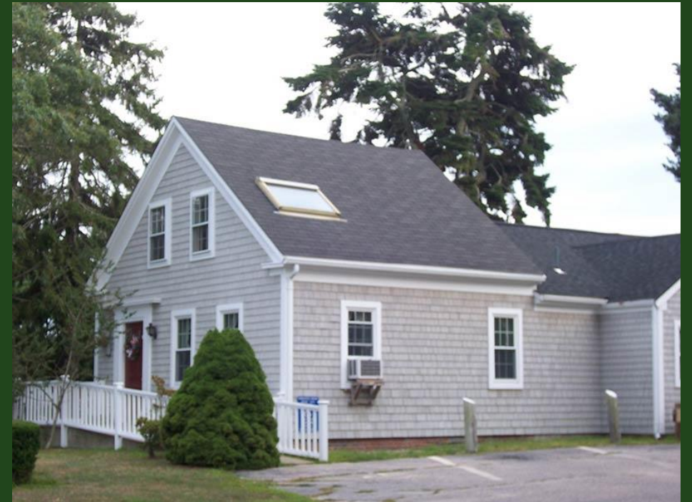
No COA is required for a skylight not visible from a public street.
