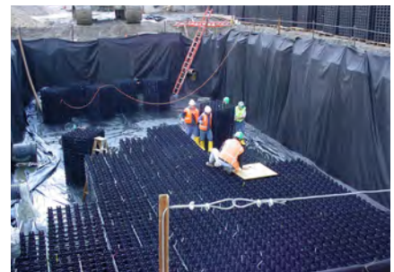
Below ground retention
