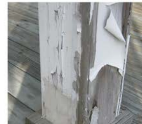
Peeling paint should be removed, the underlying surface prepared, and new paint applied according to manufacturer's recommendations to protect exterior woodwork from moisture, insects, and solar effects
