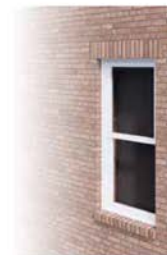
Brick lintels can be as simple as a single soldier course supported by a steel lintel behind. Other appropriate brick lintels include arches and jack arches. Brick sills are typically a single sloped rowlock.
