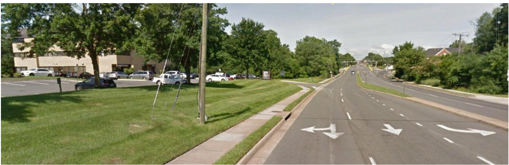
Photo of inadequate separation between travel lane and sidewalk – Located along Elden Street
