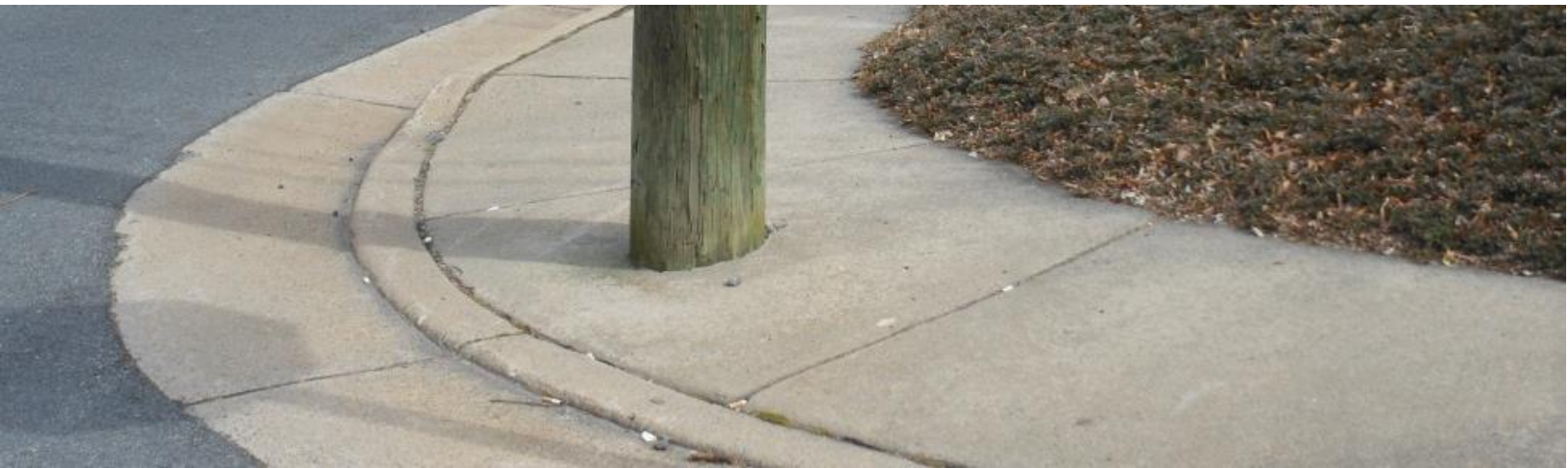
Photo of telephone pole within sidewalk ramp – Located at Elden Street and School Street
