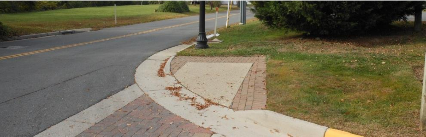
Photo of ramp of missing sidewalk – Located at Monroe Street near First Baptist Church
